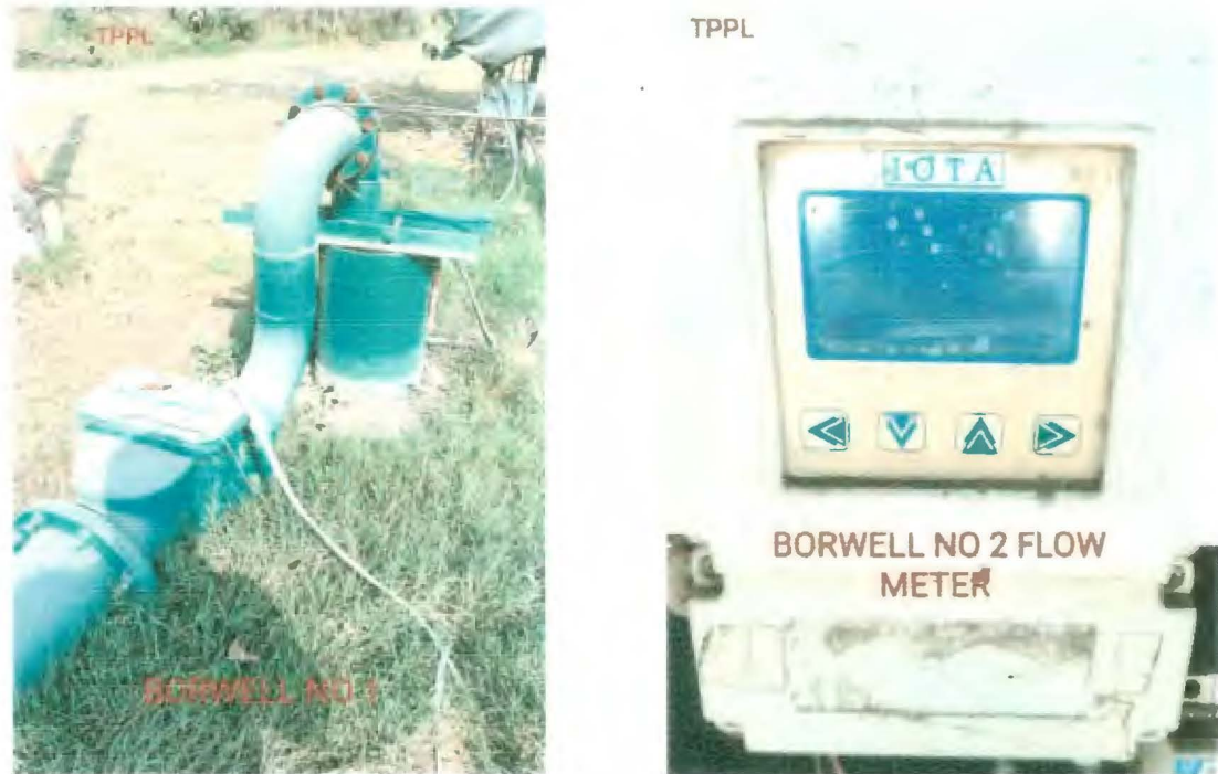
Fig. - 2: Borewell Flow Meter at Tehri Pulp and Paper Limited, Unit-2
